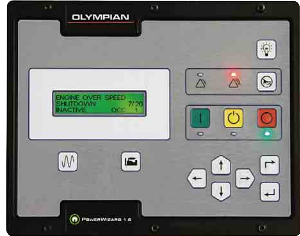
PowerWizard 1.0 kontrol panel
